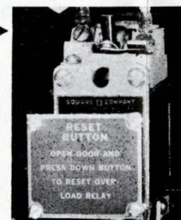
In Control Panel.
